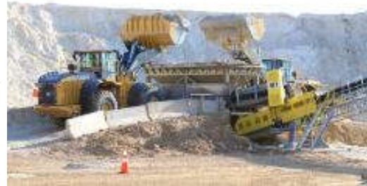
Conveyer Belt to On-site Wet Plant
