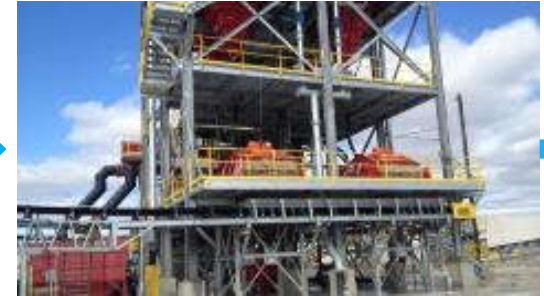
Wet Plant Cleans and Sorts
